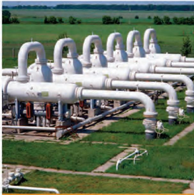
Gas Processing & Transmission
